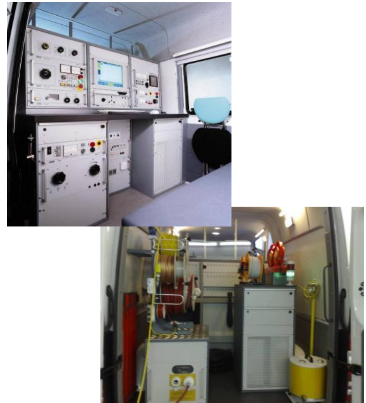
Cable fault location + VLF testing and TD + PD diagnostics
