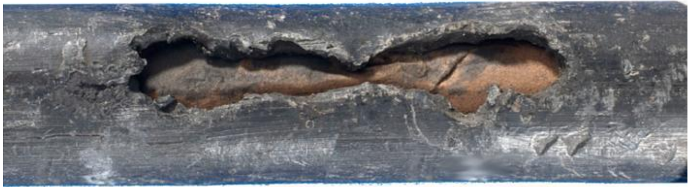
Corrosion of a lead coated PILC
